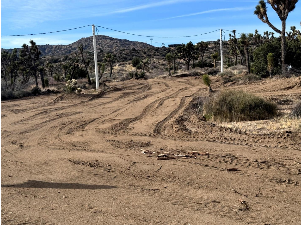
Figure 3. Recent installation of infrastructure and surface disturbance of the Cielo property held in trust by the Bureau of Indian Affairs for the Twentynine Palms Band of Mission Indians.
